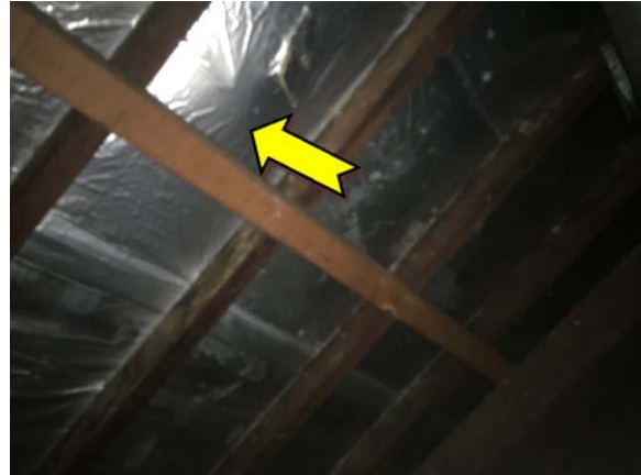
Photo 14. Interior, art room, roof space, under side of roof – suspected SMF sarking insulation material.
