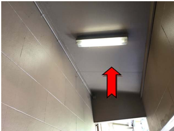
Photo 3. Exterior, ground level, east side of building, awning – suspected asbestos-containing fibre cement sheeting.
