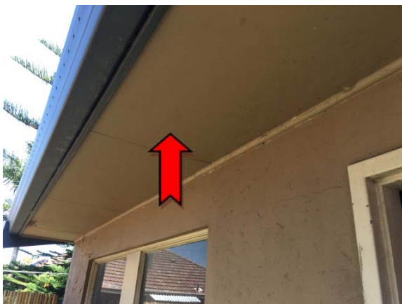
Photo 5. Exterior, ground level, toy store, east side, eaves – suspected asbestos-containing fibre cement sheeting.
