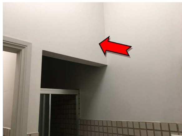
Photo 6. Interior, level one, staff room, toilet, east, south & dividing walls – asbestos-containing fibre cement sheeting.
