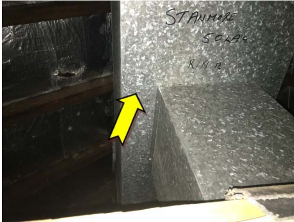
Photo 13. Interior, art room, roof space, air handling ductwork – suspected SMF internal insulation material.
