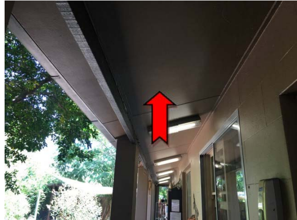
Photo 2. Exterior, ground level, south side of building, west end, awning – asbestos-containing fibre cement sheeting.
