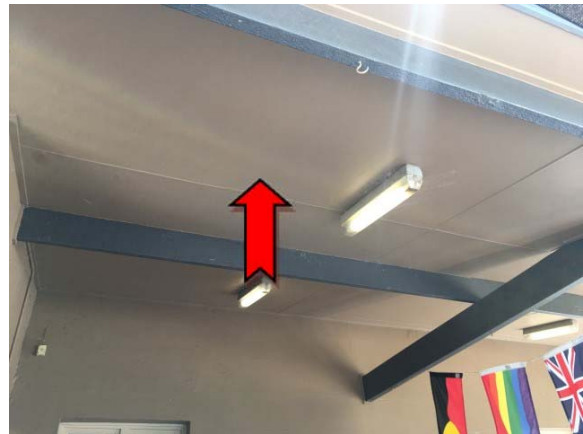
Photo 4. Exterior, ground level, east verandah, awning – suspected asbestos-containing fibre cement sheeting.
