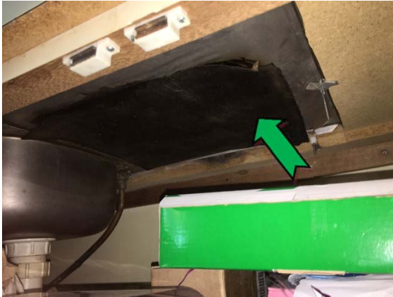
Photo 7. Interior, level one, art room, beneath sink, sink pad – non asbestos-containing bituminous membrane.
