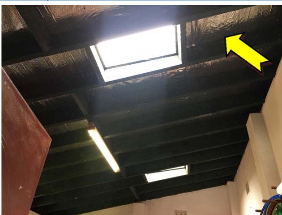
Photo 11. Exterior, ground level, toy store, under side of roof – suspected SMF sarking insulation material.
