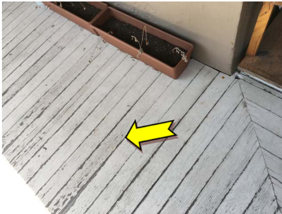
Photo 15. Exterior, level one, verandah, floor – suspected lead-containing blue upper paint systems.
