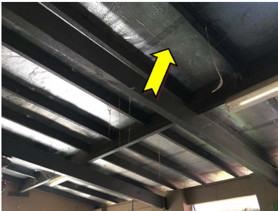
Photo 9. Exterior, ground level, play area, insulation – suspected SMF sarking insulation material.
