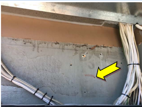
Photo 17. Exterior, ground level, inside electrical cabinet, wall – lead-containing grey upper paint systems.
