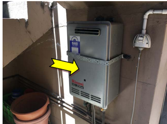
Photo 10. Exterior, ground level, west alleyway, hot water heater – suspected SMF internal insulation material.
