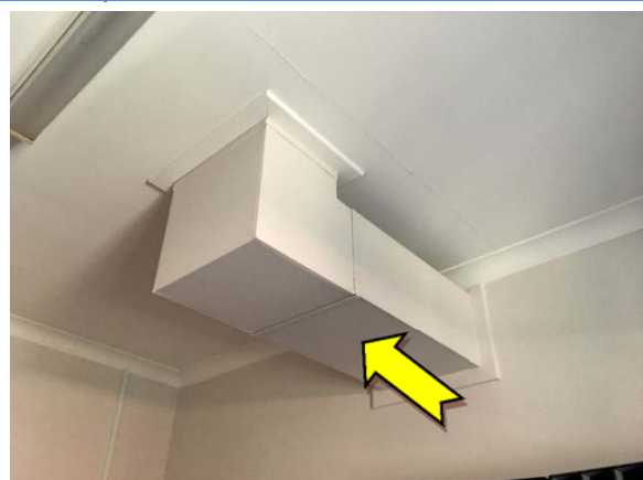
Photo 12. Interior, level one, office, air handling ductwork – suspected SMF internal insulation material.
